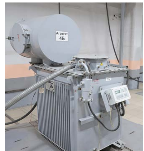
New electrostatic precipitators at West Siberian Thermal Power Plant
