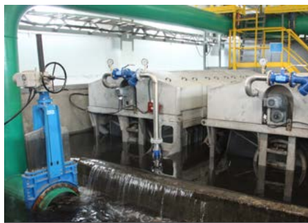
New mine water treatment facility at Raspidskaya mine
